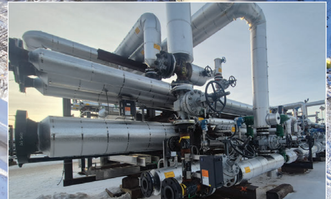
Well Pad Facilities
