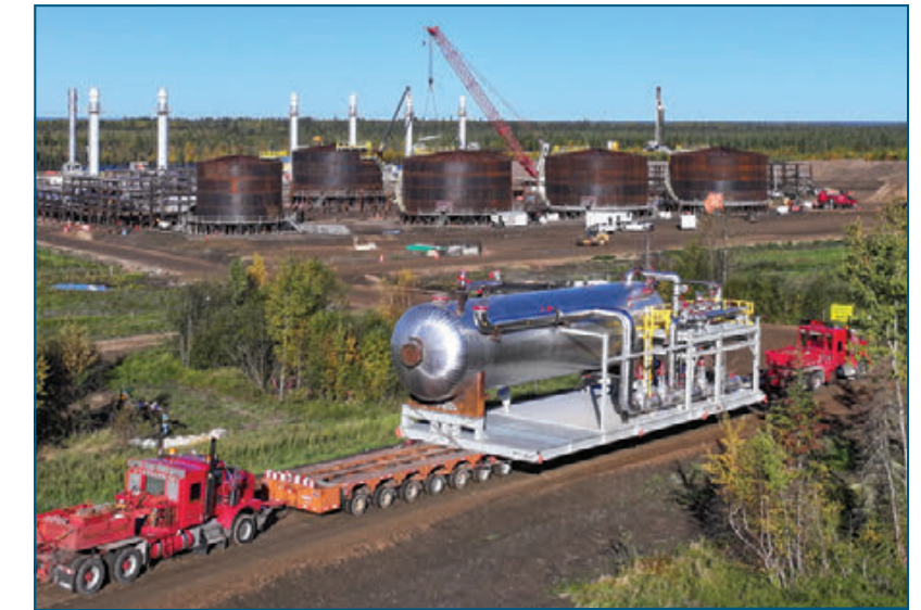
Inlet degasser at site
