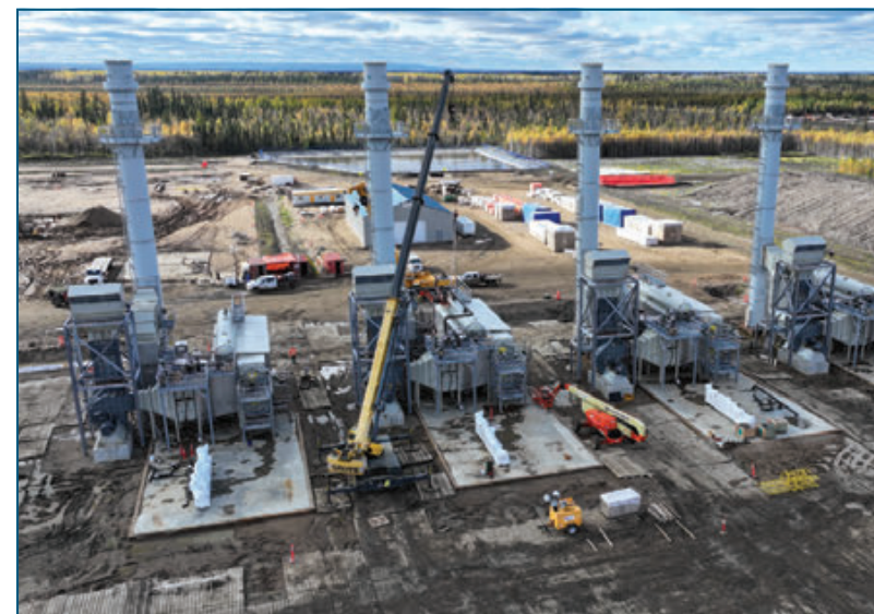
Boilers in place
