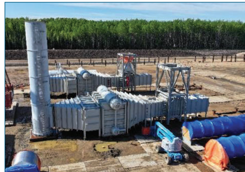
Heat recovery steam generators in place
