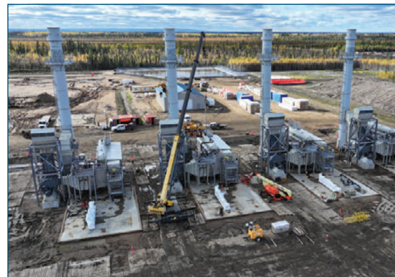
Boilers in place
