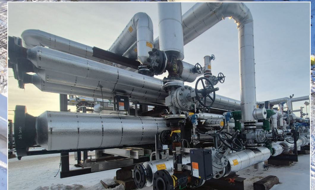
Well Pad Facilities
