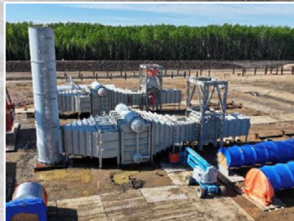
Heat recovery steam generators in place
