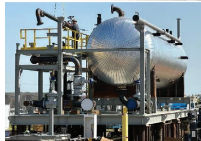
Fabrication inlet degasser
