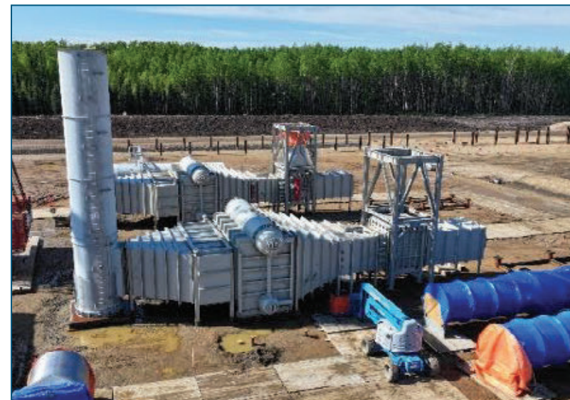
Heat recovery steam generators in place
