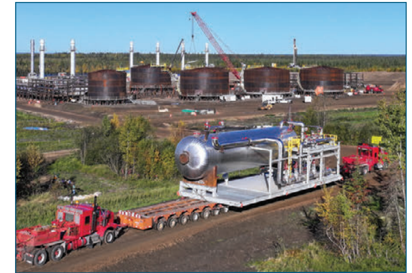
Inlet degasser at site
