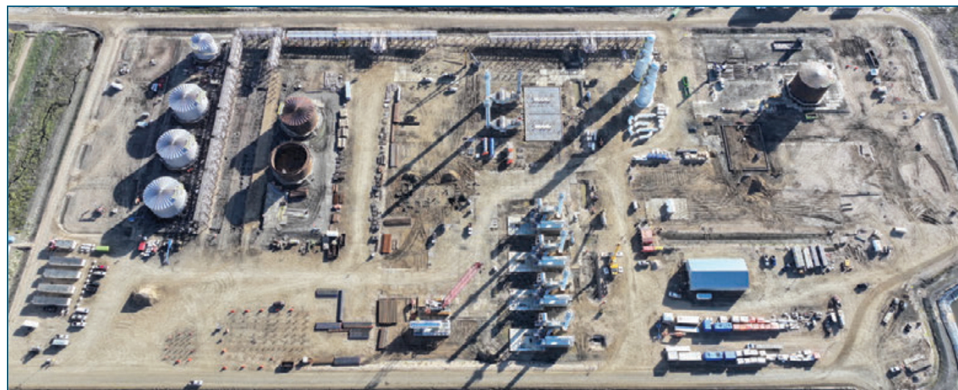
Blackrod Central Processing Facility (CPF)
